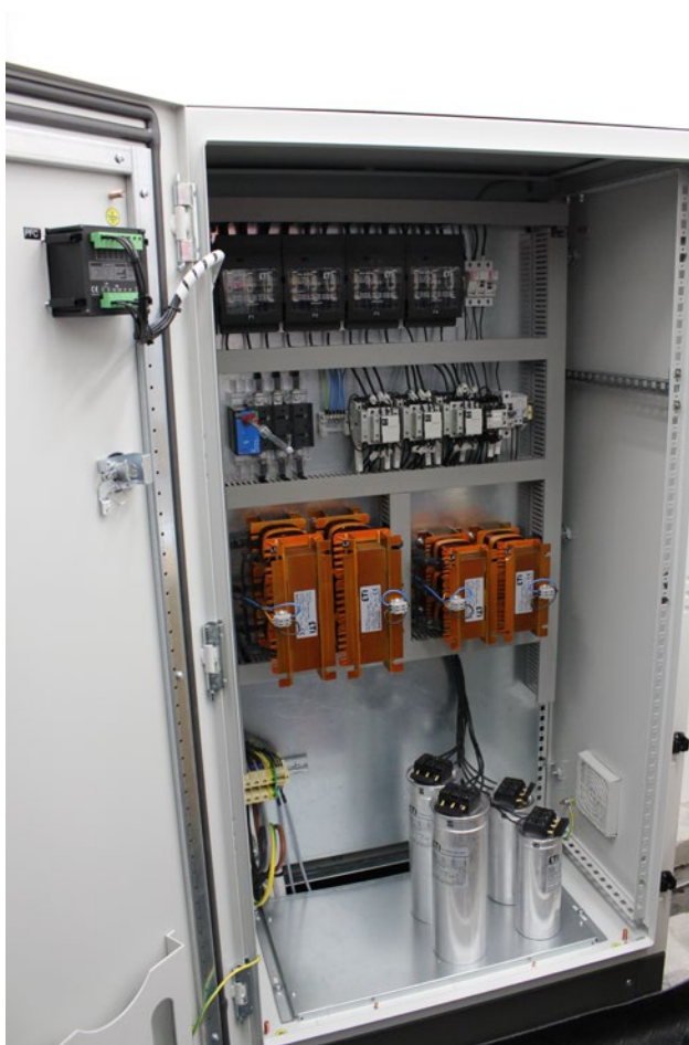
Automatic Power Factor Correction Banks
